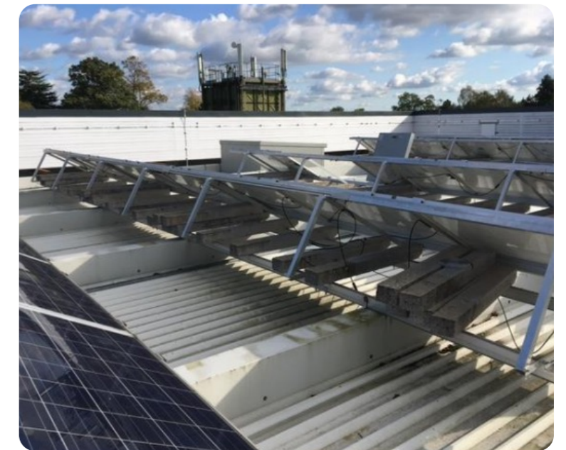
Solar PV on Support Services Building. Source SWFT Library
